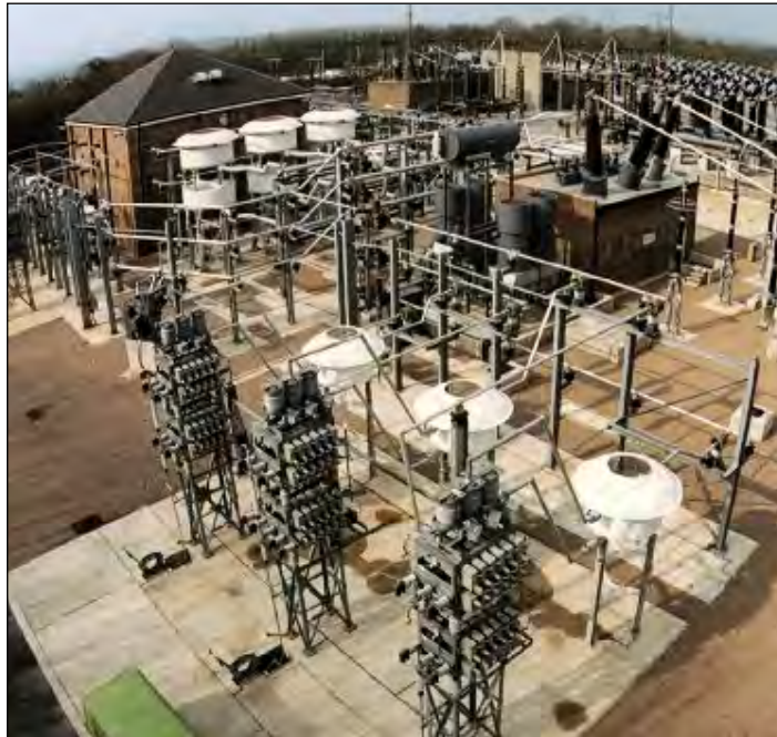
Figure 6.4.3: Typical SVC installation built in a transmission substation – rating: 225MVar
