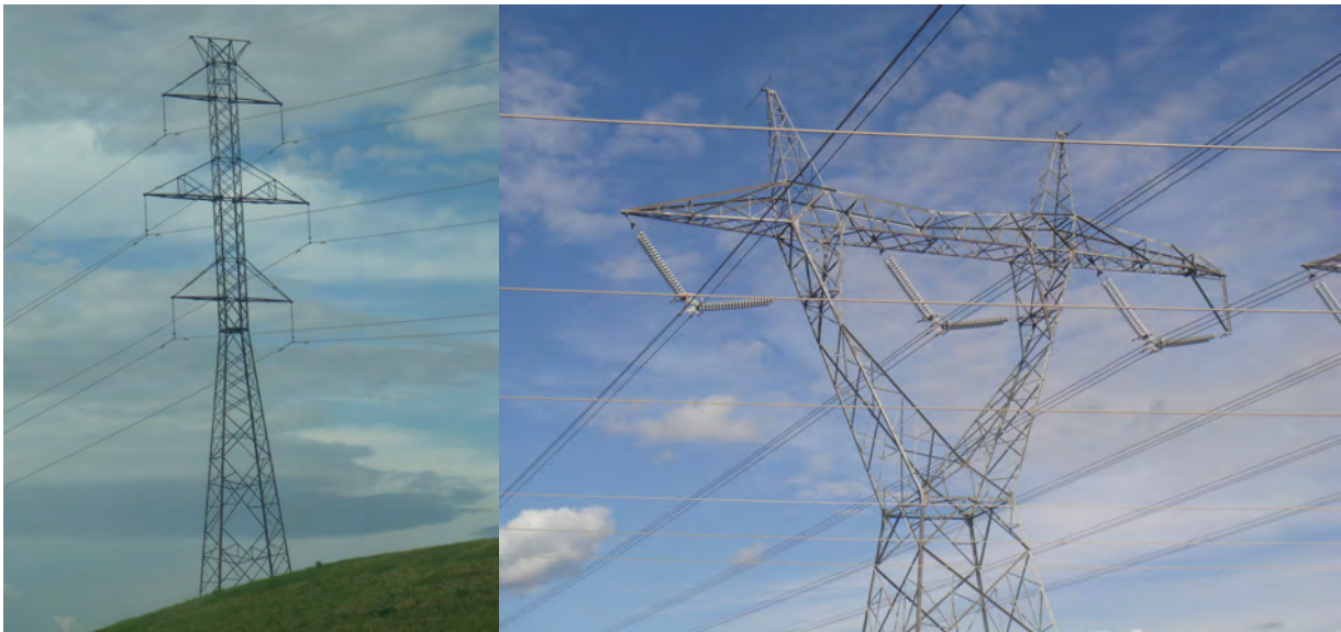
Fig. 6.2.(a) Typical 240 kV and 500 kV transmission Lines in the Edmonton area
