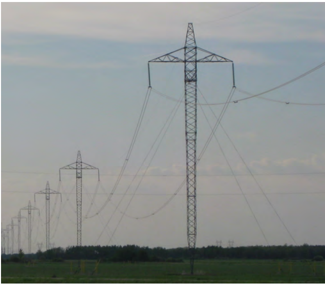
Figure 9.1.10 : Example of use of guyed masts as HVDC transmission structures. Nelson River HVDC Transmission System.
