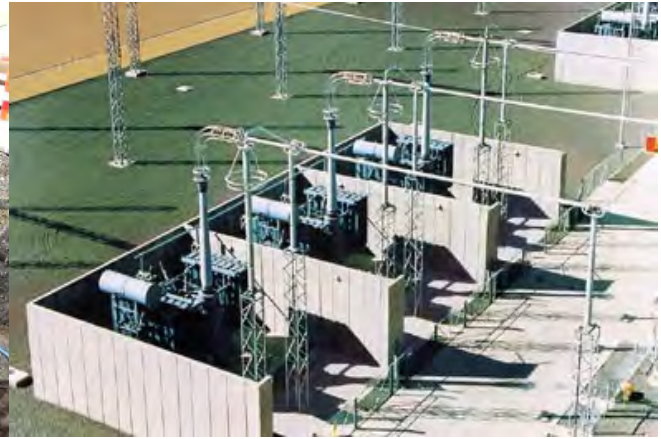
Fig. 7.8(b) Three Single Phase Shunt Reactors
