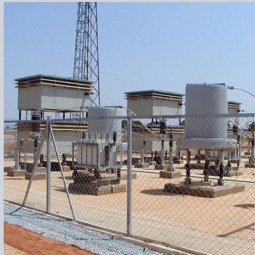
AC Harmonic Filters – Talcher Station (ESI - II)
