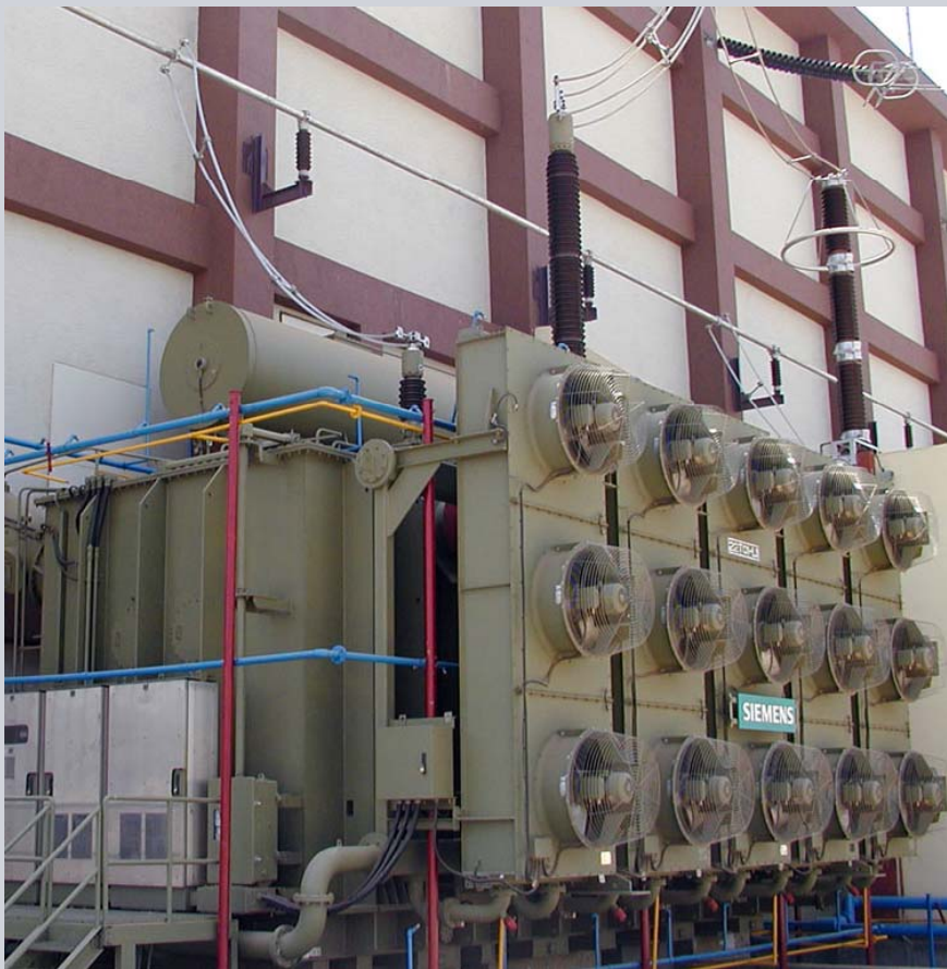
Converter Transformer and Valve Hall – Talcher Station (ESI - II)
