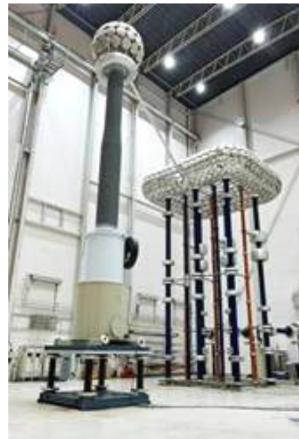
Fig 5. Testing of transformer bushing
